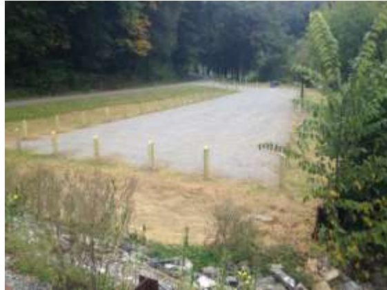
Fisherman's Paradise – Upper Parking lot stormwater diverted to swale at bottom
