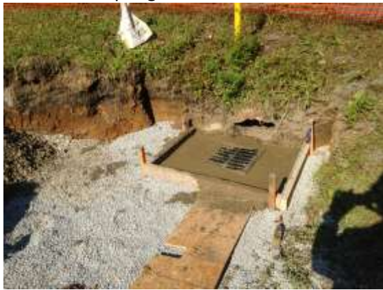
Stormwater enters grill and is piped to wetlands
