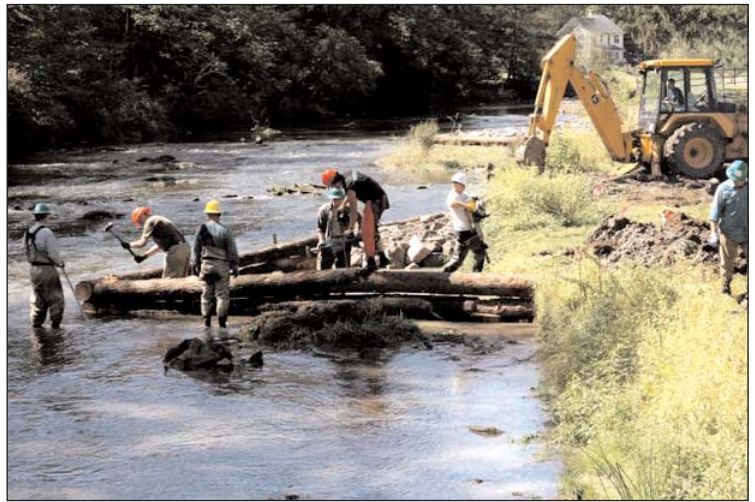
A crew installs logs at one of SCTU's previous stream improvement initiatives, the 550 Project.
